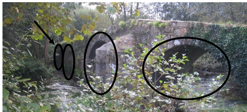
Fig.2. Side view of the Lubiáns Bridge, with its four arches highlighted by black circles. The arrow points the arch subject of deeper study due to a previous detection of moisture in it.
