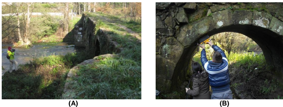
Fig.1. Thermographic survey on the first arch upstream (A) and GPR survey over the vault of the same arch (B)
